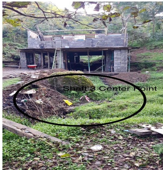
On-going construction of the house at the location of the tunnel shaft
